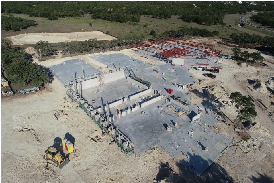
Aerial View of Slab on Grade (photo taken by Bartlett Cocke General Contractor)
